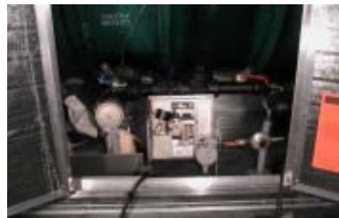
Easily accessible inlet and discharge piping.
